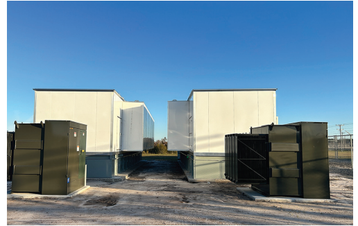
Northeast Florida is the location of two high-security prisons. Clay Electric installed these backup generators to serve both sites.
