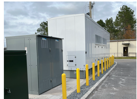
Clay Electric decided that this new backup generator was the best solution for aging equipment at a 99-bed acute-care hospital.
